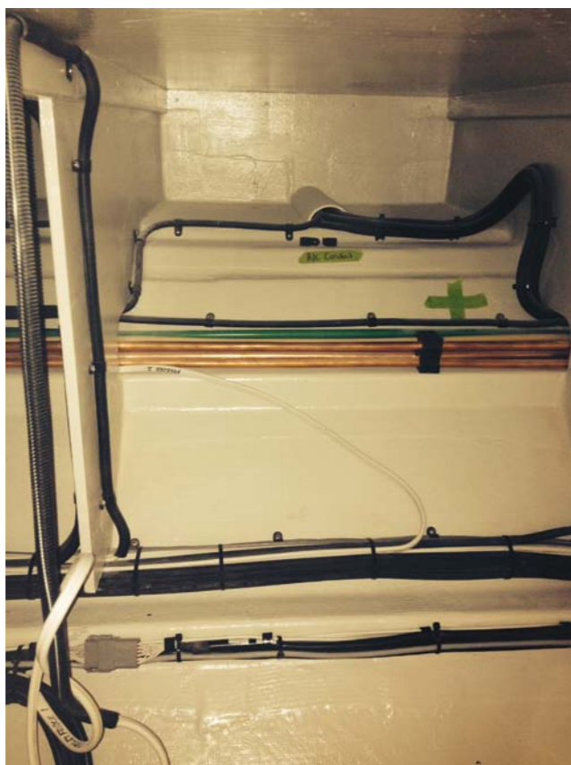
Plumbing and electrics are run down individual paths both along the hull and across the wingdeck.
